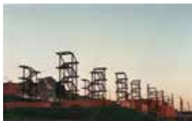
4. Construction of Mutirão Juta Nova Esperança, Usina, Sao Paulo, 1994-1999, Image © Usina CTAH
